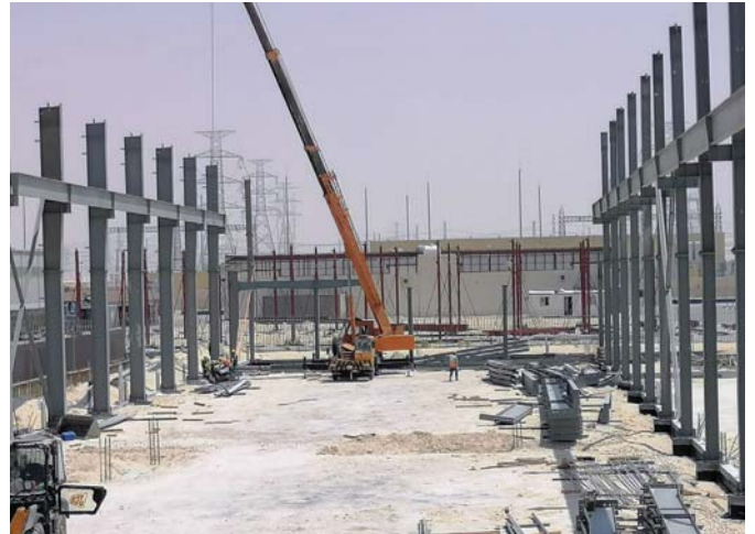
Construction work in progress at the new facility of Thejo Hatcon Industrial Services Company at MODON Industrial Area 3
