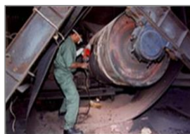
Conveyor pulley lagging (Lagging of conveyor belt pulleys)
